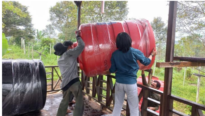
Gambar 4. Instalasi Sistem Irigasi Rainwater Harvesting (RWH)
